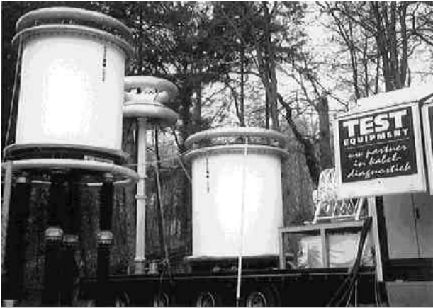
Figure 3 After-laying test of 420 kV cable with the aid of the mobile test set-up. One HV reactor and coupling capacitor standing on the trailer and the second reactor on a platform isolated for 220 kV.
